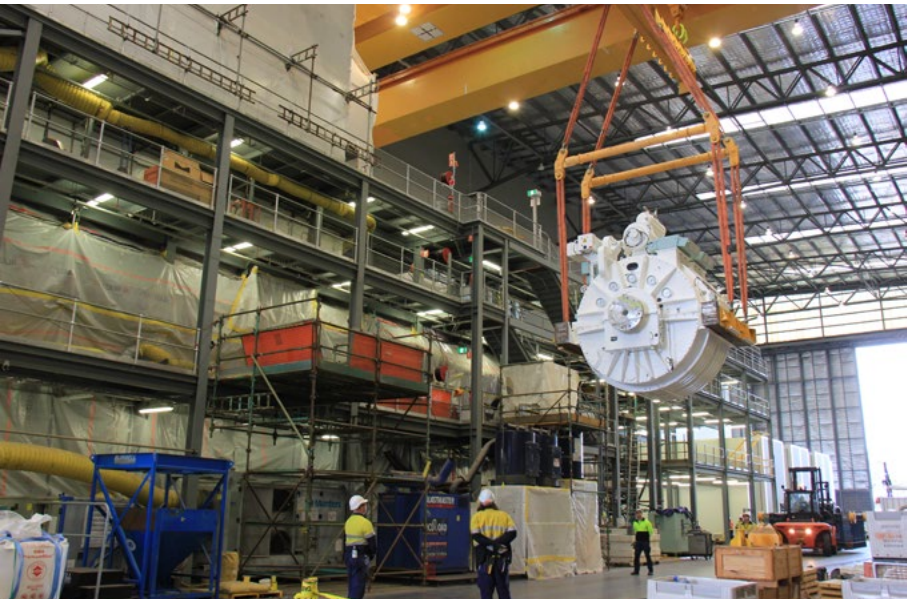
Removing the major systems from the submarine allows them to be worked on in a more spacious environment than is possible within the hull. As well, it's possible to fit already refurbished replacements, facilitating a faster turnaround by managing a stock of spares rather than delaying the return of a boat to service until its 'own' systems can be returned. (Photo courtesy ASC).
