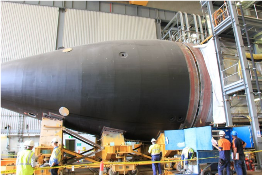
With refurbished components reinstalled, the hull can then be rejoined and welded as part of the process of returning the boat to service. (Photo courtesy ASC).
